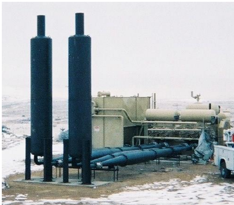
Figure 11: Expansion Pipes with a DPC-2804LE
