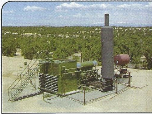
Figure 1: AJAX DPC-2803LE Package In Southwestern USA
