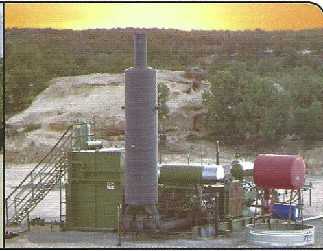
Figure 2: AJAX DPC-2803LE Package In Southwestern USA
