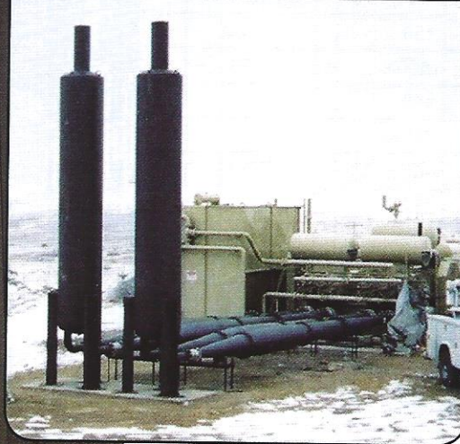
Figure 11: Expansion Pipes With A DPC-2804LE
